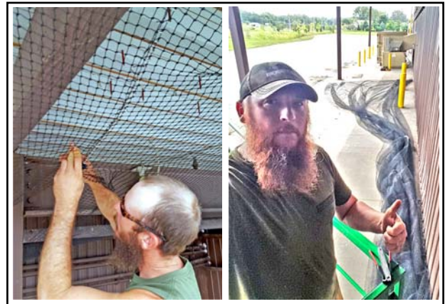
The skilled installers at River Valley Wildlife Specialists had worked with Nixalite's K-Net bird netting before. With help from Nixalite, they formed an installation plan and followed it all the way to completion with very few alterations.
